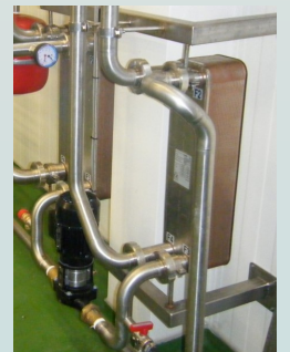
Heating with heat exchanger
