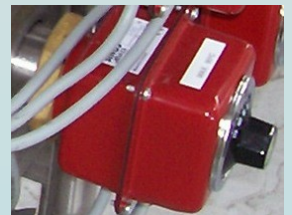
Electrical heating elements
